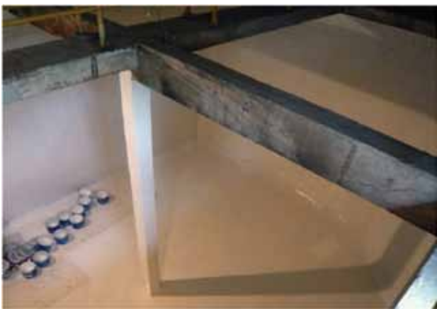
INDONESIA Sewage Treatment
